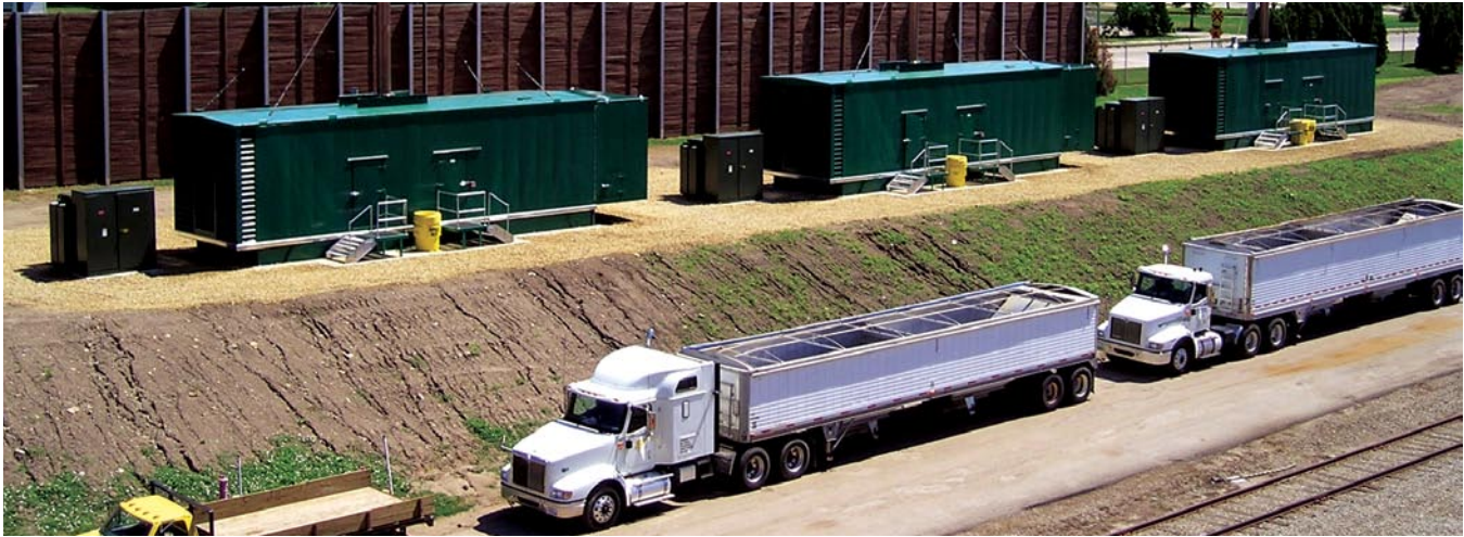
Trucks at our Austin, Minn., facility alongside generators installed as part of our energy partnership with the local utility company.
